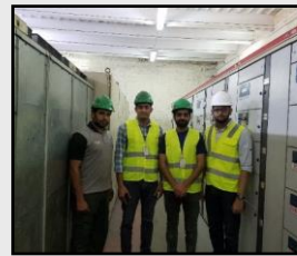
Energy Audit of Electric Panels
