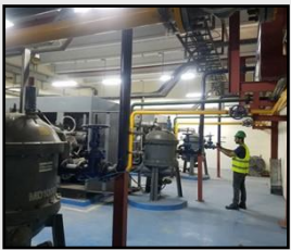
Energy Audit of Compressors
