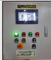
Pump Testing Control Panel
